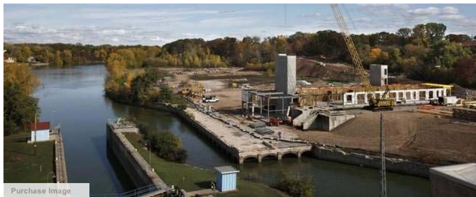
Workers from C.D. Smith Construction of Fond du Lac work on the newest riverfront development project under way along the Fox River and College Avenue bridge in Appleton. The 32-unit apartment building is called 'Evergreen.' / Sharon Cekada/Post-Crescent Media
